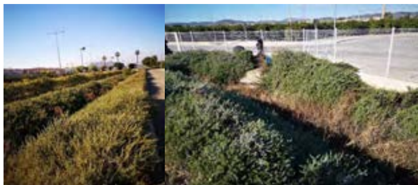
Figure 13 Current state of the vegetated swales under study. Left: North Roadway swale, right: Sport Area swale
