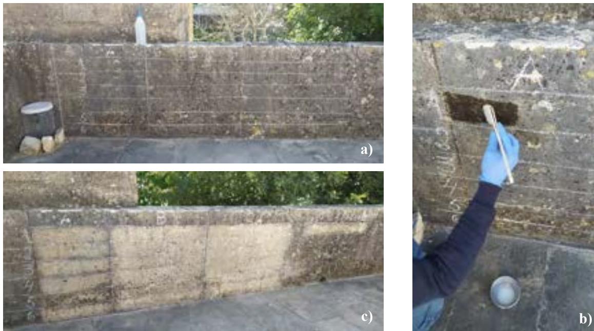
Figure 2. Pictures of the tested site on the inner face of the parapet of the Terrace of the Count. (a) Rectangular tested areas for the application of one (A), two (B) and three coats (C) of biocides and controls specifically: Tm (1), Mp (2), Fv (3), Rv (4), SDS (5), Biotin T (6), water. (b) Application of the biocides and controls in the first week. (c) After cleaning, five weeks after the beginning of the application of the first coat.
